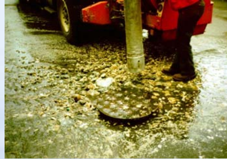
SSO from excessive flows
