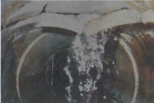
Infiltration due to pipe break
