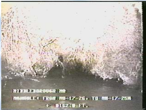
Roots blocking pipe
