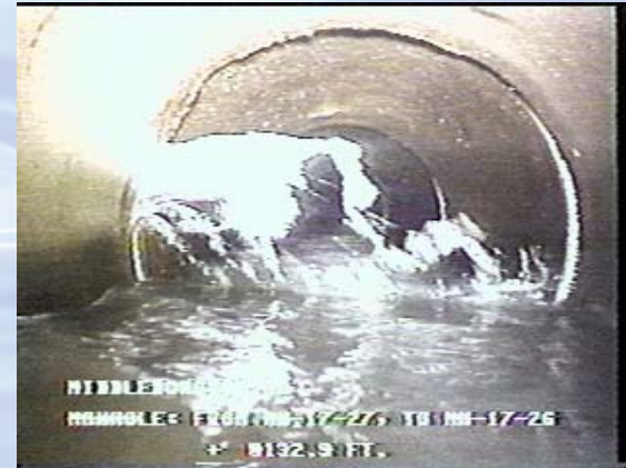
Infiltration due to leaking joint
